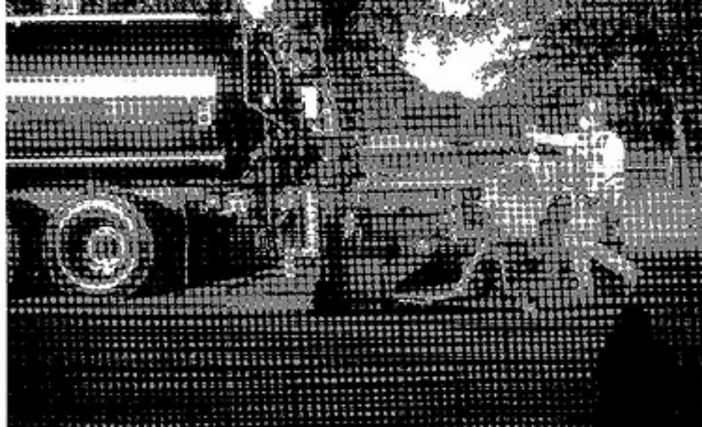
The telescoping paving fabric installation machine places the paving fabric into the oil as the truck spreads the oil.
