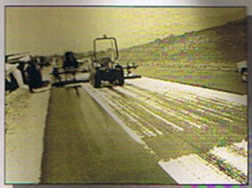
Thin fabric doesn't hold tack coat as easily, resulting in bleed through, which can be hazardous to workers and equipment.
